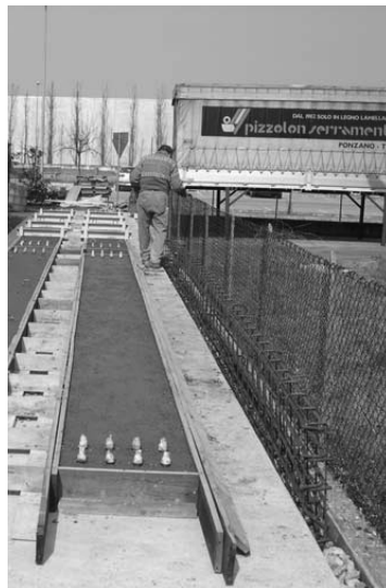
Figure 1 – Field tests on restrained drying shrinkage of concrete slabs (8 m long, 400 mm wide and 60 mm thick).
